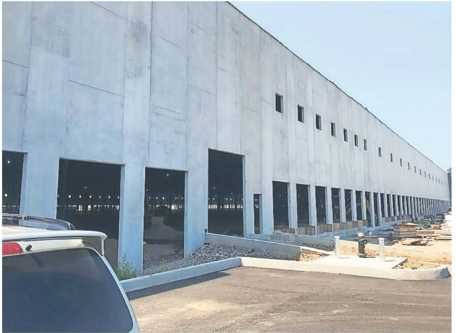
The first warehouse — a 975,000-square-foot building the size of 27 football fields — in the new 200-acre Matrix Global Logistics Park Staten Island is expected to be complete in September. Tracey Porpora, Staten Island Advance
